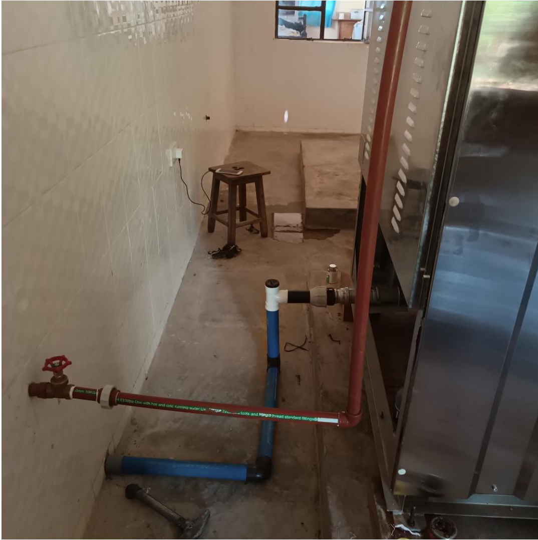
Fig 10: The in and out water system already installed
