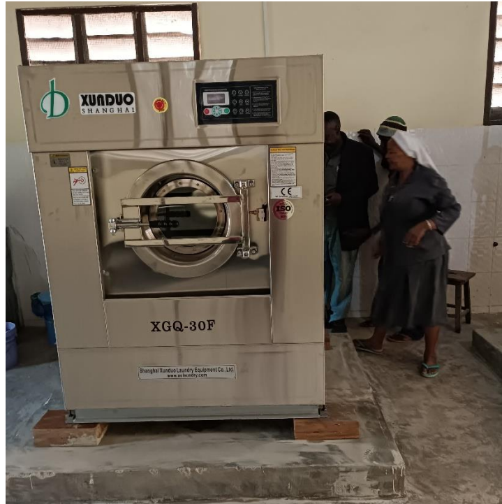
Fig 7: The machine already kept in its permanent base and tighten by bolts
