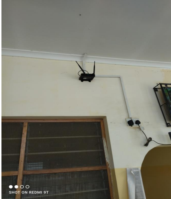
WIRELESS ACCESS POINT AT OPD BUILDING
