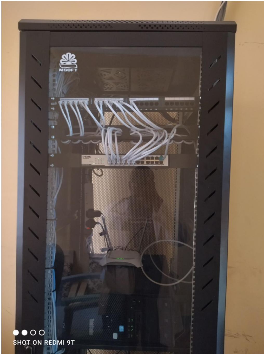
SERVER IN THE RACK CABINET
