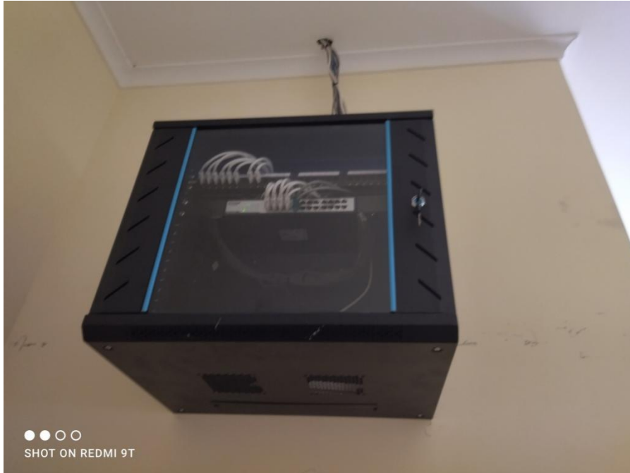
24 PORT SWITCH FOR MINOR THEATRE BUILDING
