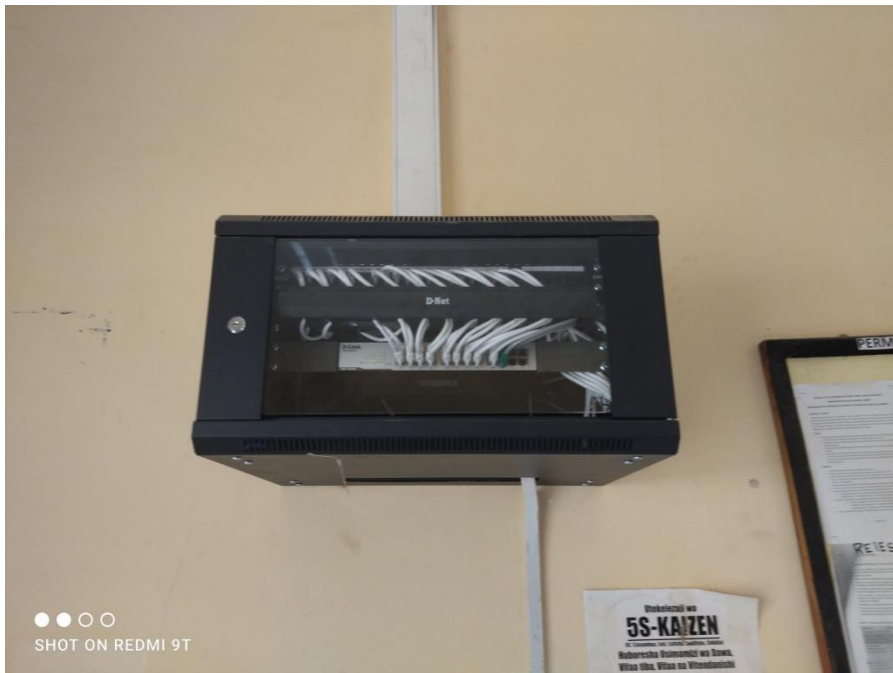
24 PORT SWITCH FOR OPD BUILDING
