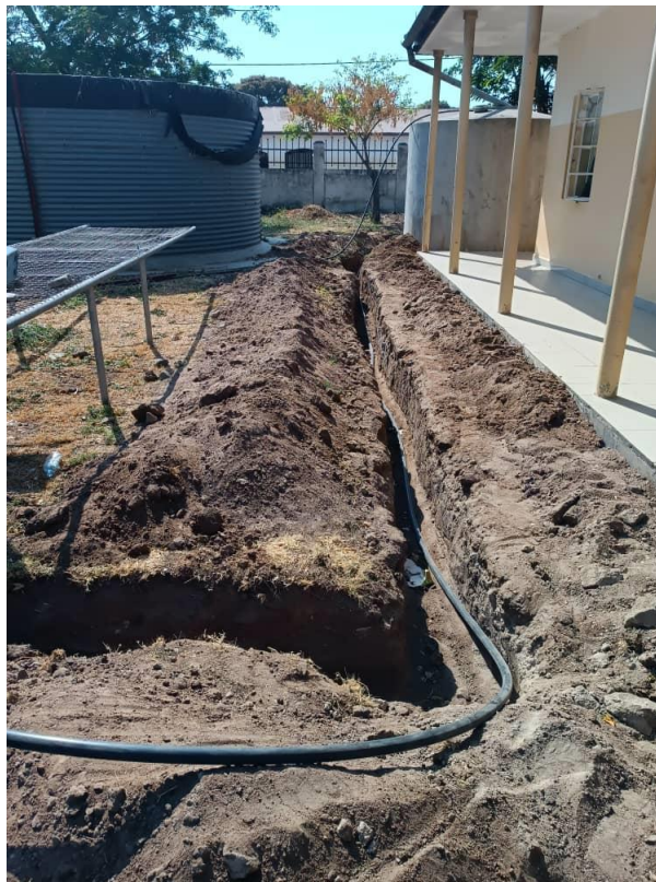
Fig 11: pipe connecting the water from the big underground tank and from ziwa Victoria source to a tower
