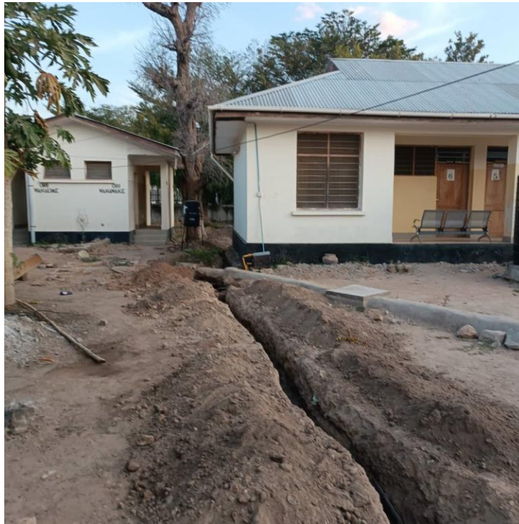
Fig 6: Trenches for laying pipes from the big underground tank to a tower where 10,000 litres tank will be kept.
