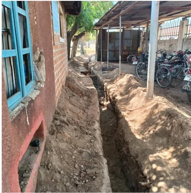
Fig 8: Trenches for laying pipes from the big underground tank passing near the minor theatre building to a tower where 10,000 litres tank will be kept.
