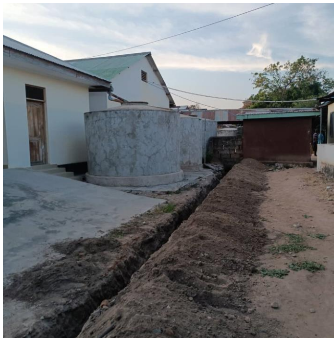
Fig 9: Trenches for laying pipes from the big underground tank passing near the laboratory and OPD building to a tower where 10,000 litres tank will be kept
