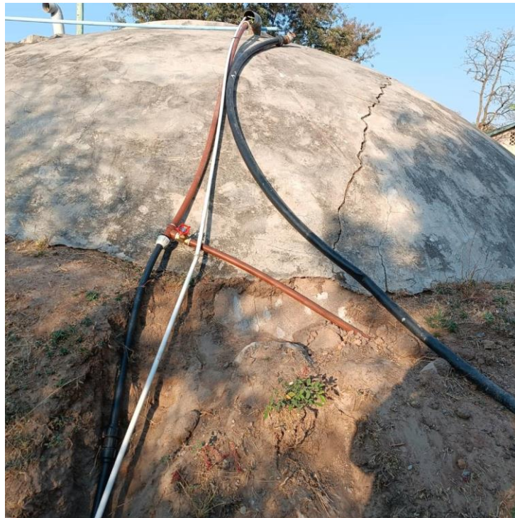
Fig 13: A big underground tank whereby the submersible pump has been kept
