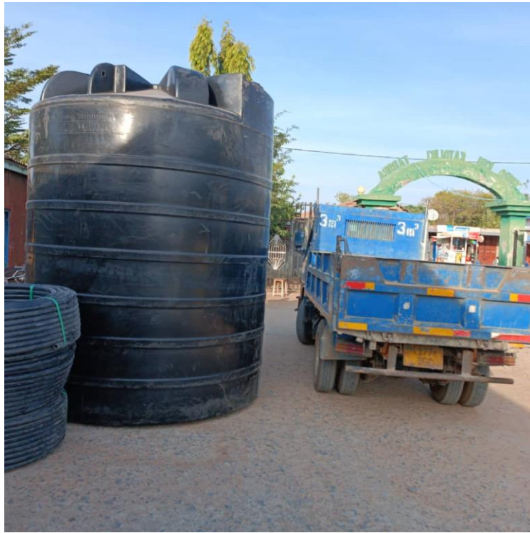
Fig 2: A 10,000litres tank with some pipes
