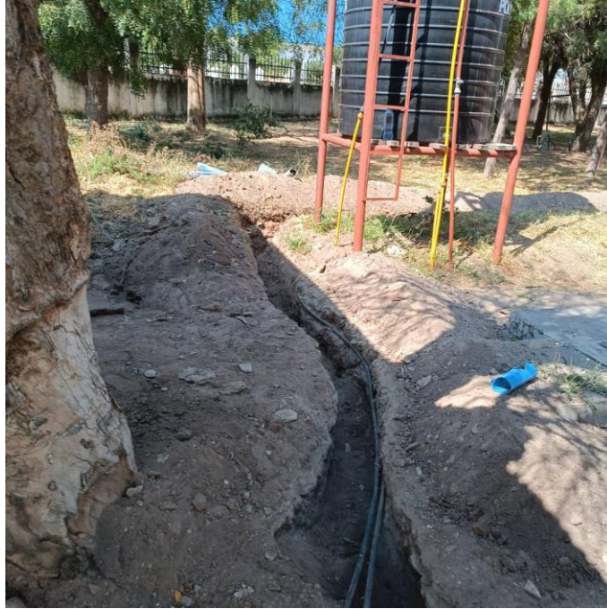
Fig 10: Trenches for laying pipes from the big underground tank passing near male ward to a tower where 10,000 litres tank will be kept
